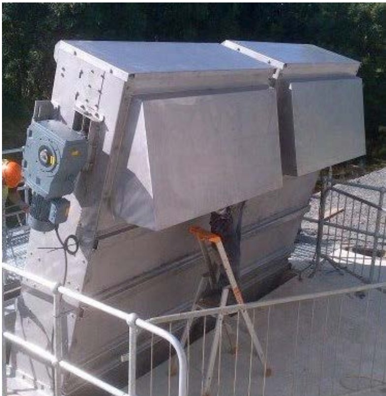
Discharge chutes from dual CBS screens
