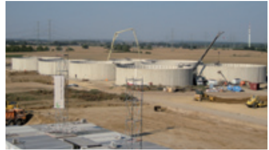
A total of five modules produce 10.000 m 3 biogas.
