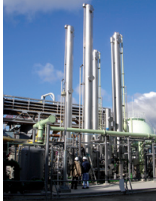
A special process is used to convert the biogas to biomethane.
